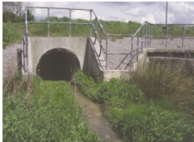
D2a Culvert – all are recorded as 'major' structures. When channel modification records 'CV', and it is impossible to see the bed and banks clearly, all other channel characteristics should be recorded as 'NK' or 'NV'.
