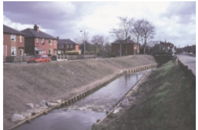
I6b Reinforced bank – toe only; reinforcement is wood-piling. Note also bed and banks have been resectioned, and a series of low weirs installed.
