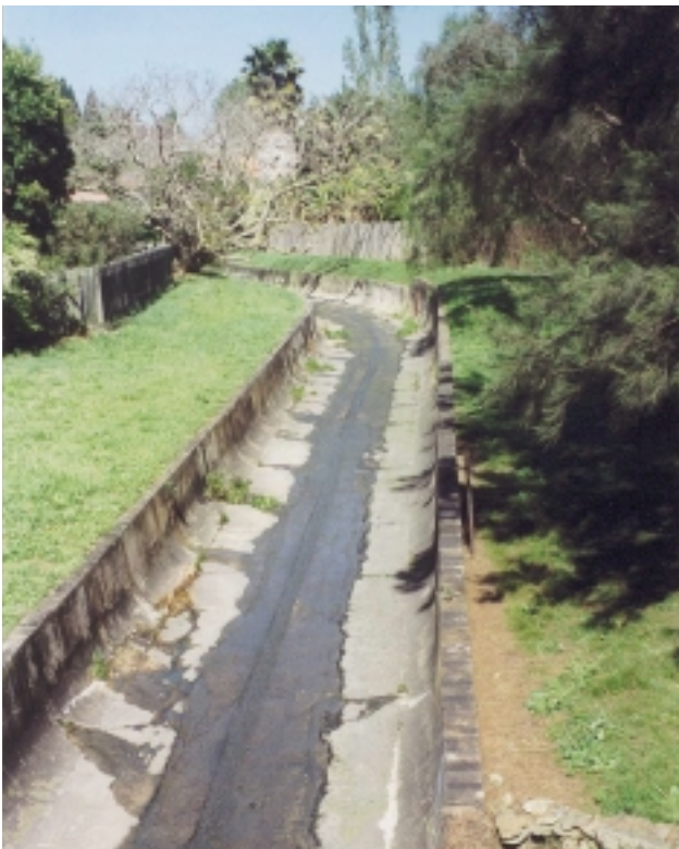
E4Ja Artificial channel substrate – both bed and banks artificial. See also D5a,b, E1La.
