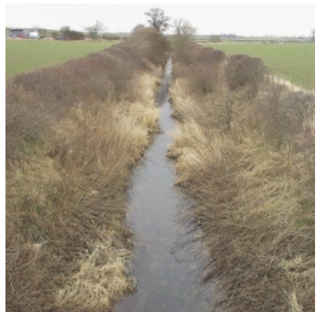
D7a An obviously realigned and over-deepened channel. Note hedge at the top of the bank that should be recorded as complex banktop vegetation structure.
