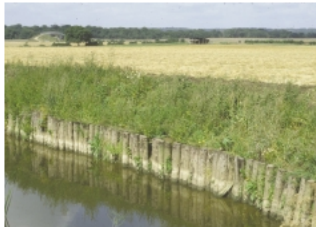
E1Jb Wood piling bank material – vertical poles below resectioned bank and arable (tilled) land-use in background.
