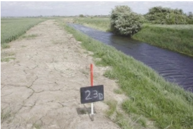
P2a Evidence of recent management – silt dredging. See E2Aa for bank mowing.
