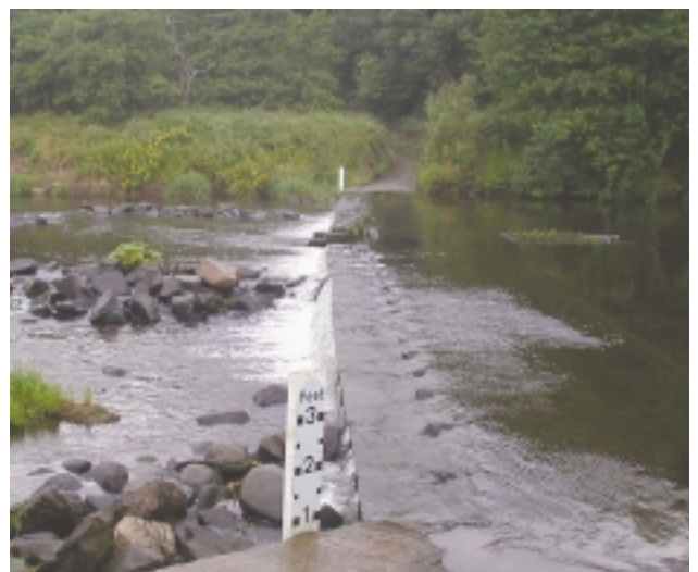
D5a Major ford – both the bed and banks are made of artificial material, and there is obvious ponding of water upstream. See also D3f.
