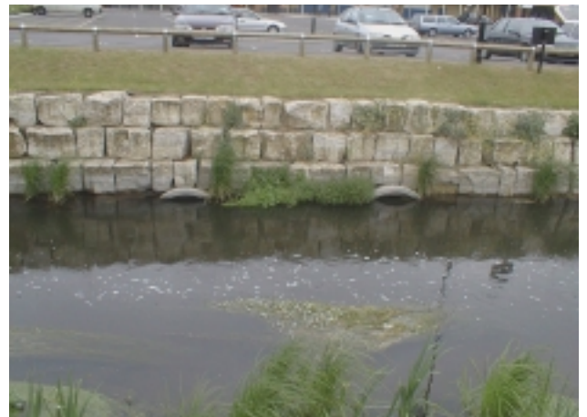
E1Mb Rip-rap bank material; placed (but not cemented), square, blocks. Note under-water 'pipes' for fish shelter (note in Section P).
