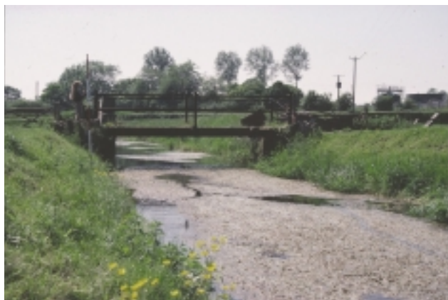
Na Realigned channel choked with submerged aquatic vegetation. Note minor bridge. See also A1b. Do not record 'channel choked' when just free-floating vegetation (see A3b).
