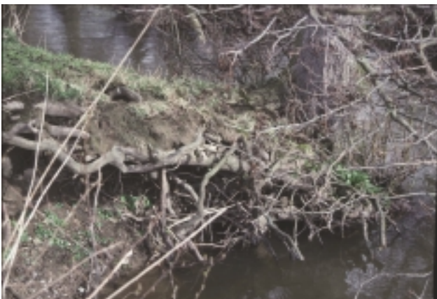
J9a Exposed bankside roots - forearm-sized roots and branches with associated cavities.
