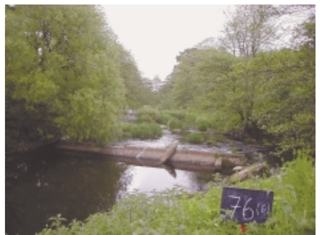
D6b This collapsed weir is recorded as a major deflector as it extends >20% across the channel.
