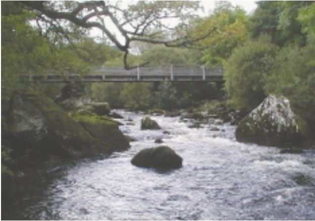
D3e Minor bridge – pipelines crossing rivers, if lacking central piers, are recorded as minor bridges. See also Na. Note exposed boulders and broken standing waves.
