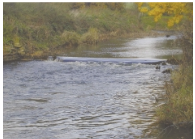
D9a Is water impounded by weir/dam? Photo shows water artificially impounded behind a shallow weir structure. See also D1b,c, D5a.
