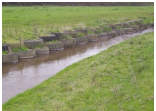
E1Nd Tipped debris – this category includes tyres, old cars, builders waste, and other materials considered as 'waste'. Record also as reinforced (RI).
