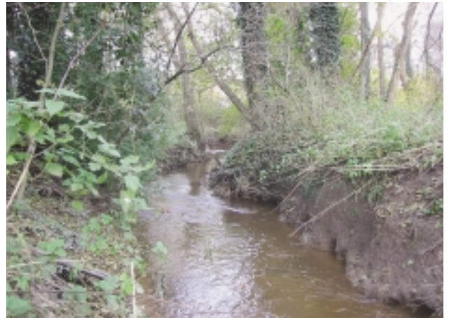
E3Bb Stable cliff – example of clay bank that is stable, but has little or no vegetation.
