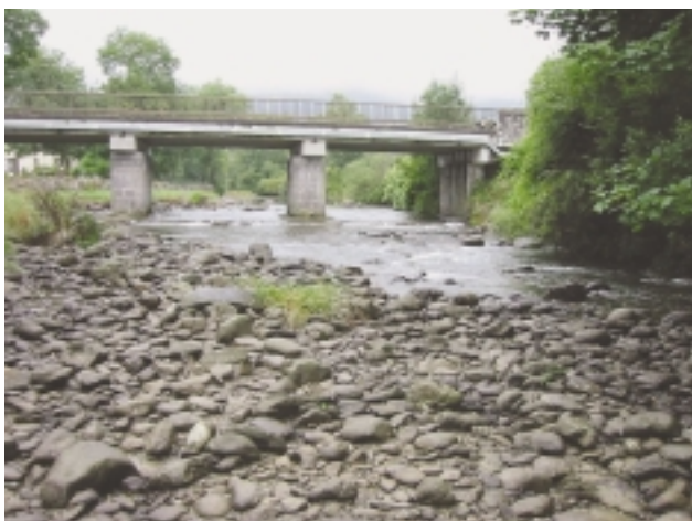
D3a Major bridge – all bridges with central piers are classed as 'major'. Note importance of photographs to show size of piers, and degree of associated bed armouring. Classic cobble channel substrate exposed in foreground. See also D5b.
