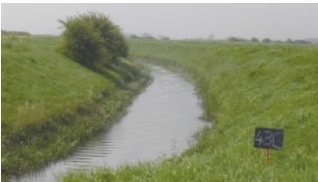
E6e Resectioned bank – this example shows river with few trees, very even gradients to the banks, and with the banktop width <4 times the banktop height indicating both deepening and resectioning.
