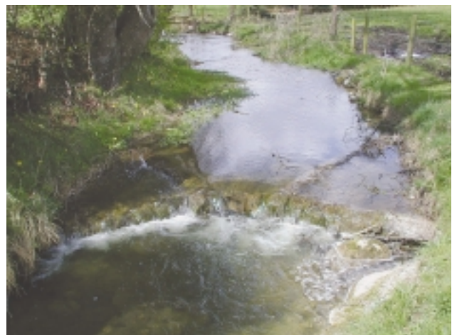
D1f Intermediate weir – wooden log construction, and water can leak through gaps.
