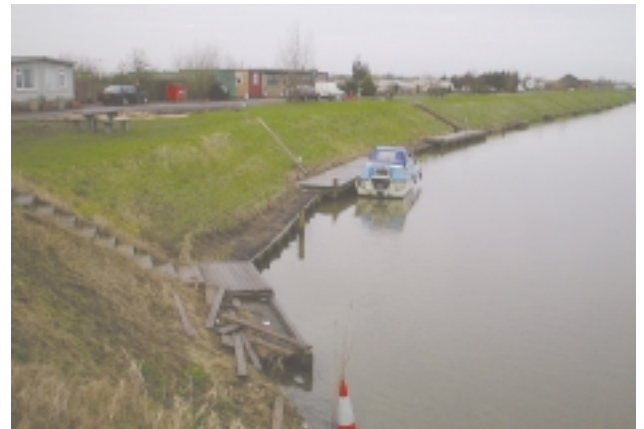
D6f Other artificial features – boat moorings. These extend 10-25m along the bank, so are classed as 'intermediate'.
