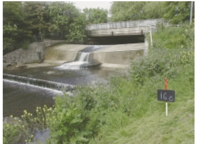
D1d Major weir/sluice – example of a complex weir structure used for measuring flow. Note also an intermediate bridge.
