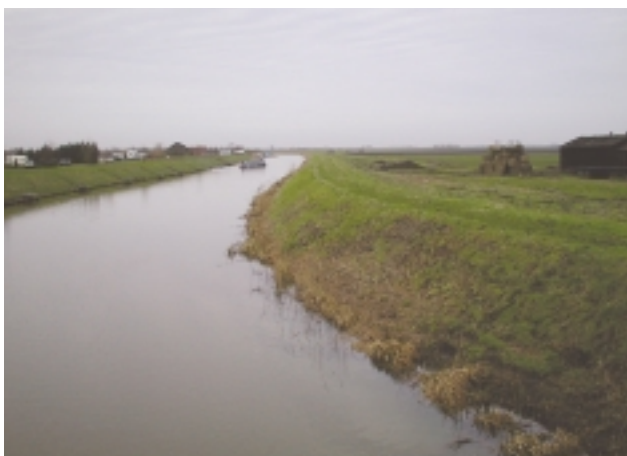
E2Da Embanked - note the earth embankment is placed on top of the natural bank (cf. set-back embankment, Section I).
