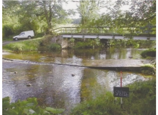
D3f Minor bridge – bridge lacks in-channel supports and has bank abutments <10m wide. Note major ford in fore-ground.
