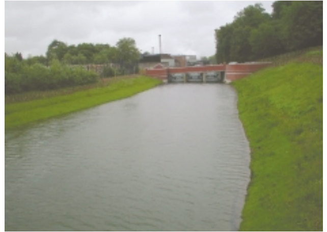
E2Ab Resectioned (reprofiled) bank – tell-tale even (trapezoidal) slope of newly resectioned bank.
