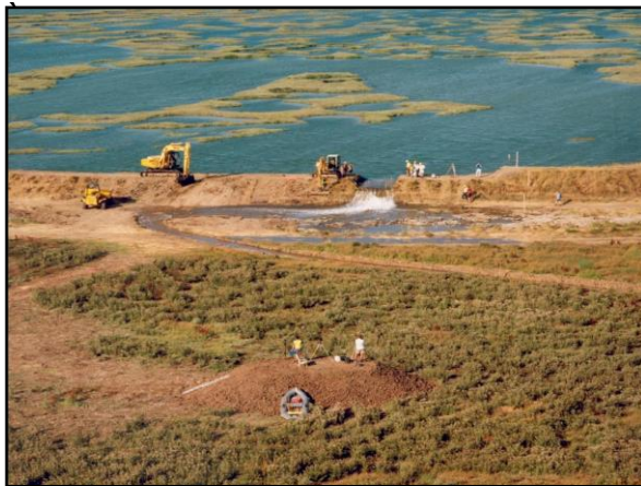
The sea wall at Tollesbury, Essex, was breached in 1995 to enable saltmarsh restoration.
